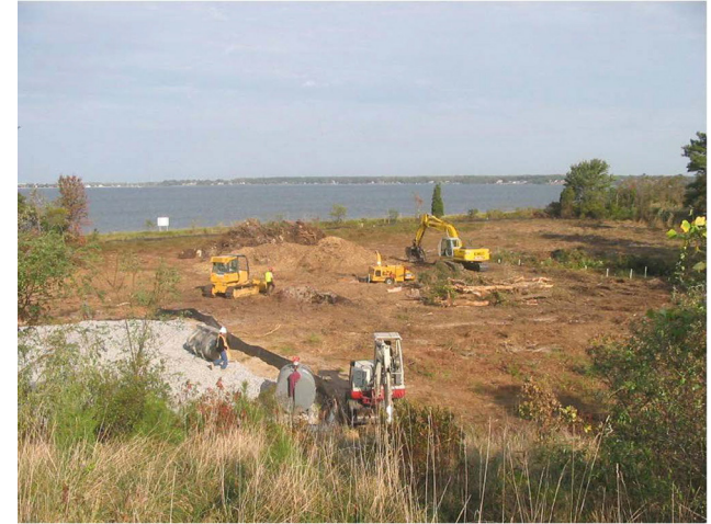
Environmental restoration work in 2007 to remove lead-contaminated soil from a closed rifle range (Operable Unit 2-Area E) at NAS Patuxent River.
